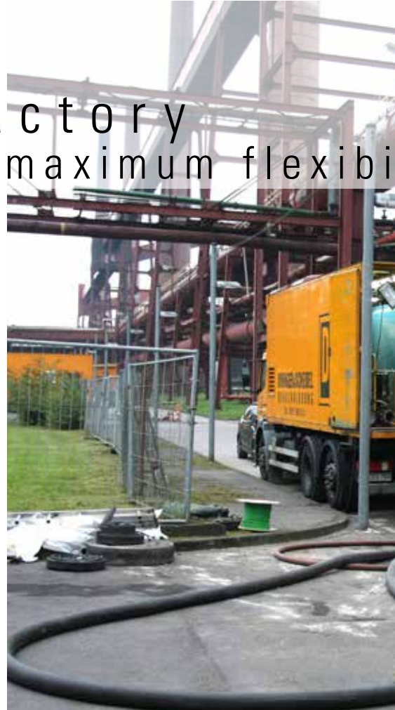
Besides the material truck, site accommodation wagon and vehicles with the heating system, an inversion tower and a conveyor belt are part of the site facilities
